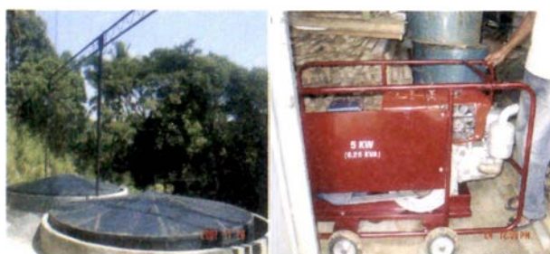
Digesters for waste handling and an Electrical generator established for the Pathdumbara Pradeshiya Sabah
